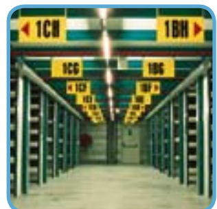
Identification on corridors and racks
